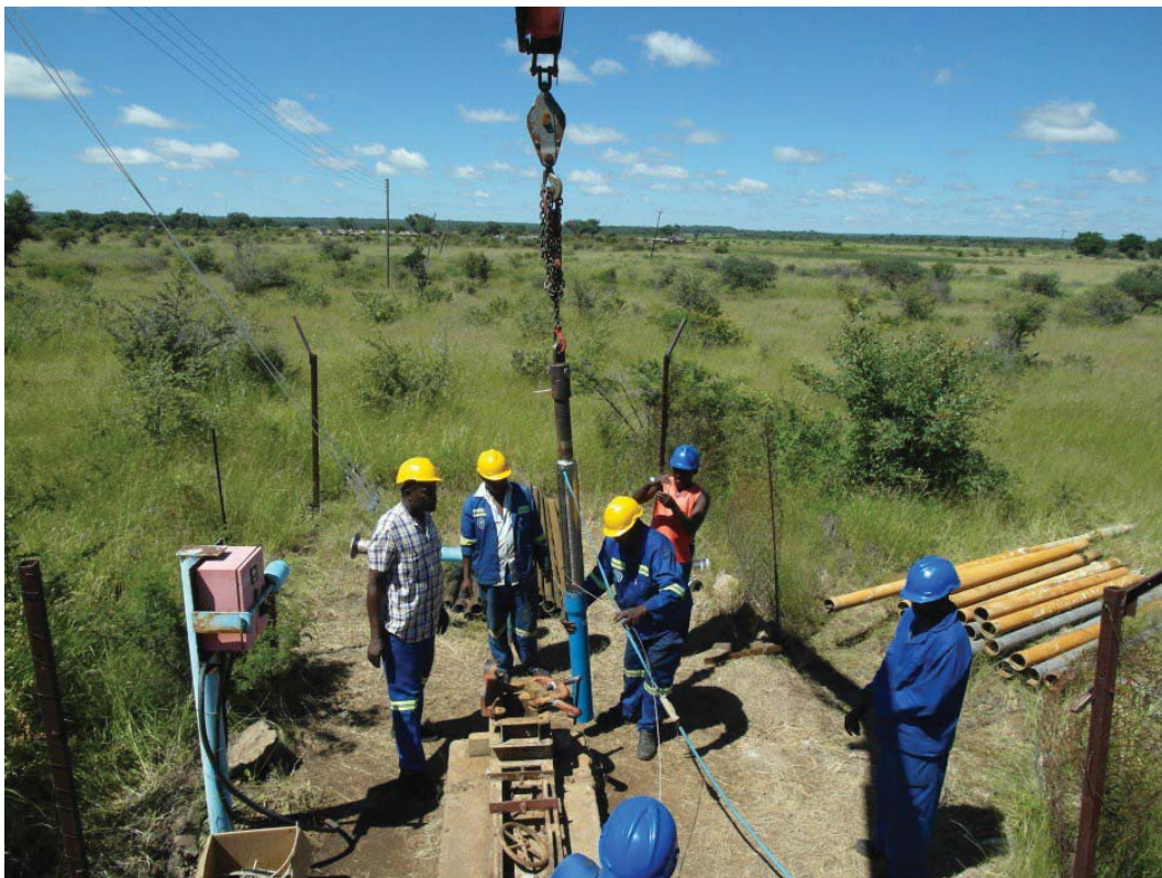
Figure 10: Installing a submersible pump in borehole 64 in the Nyamandhlovu area for pumping tests (photo credit Hans Beekman)
