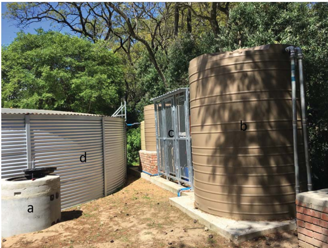
Figure 1: Groundwater supply system (a) borehole equipped with submersible pump (b) raw water tank (c) water treatment (d) water storage tank.
